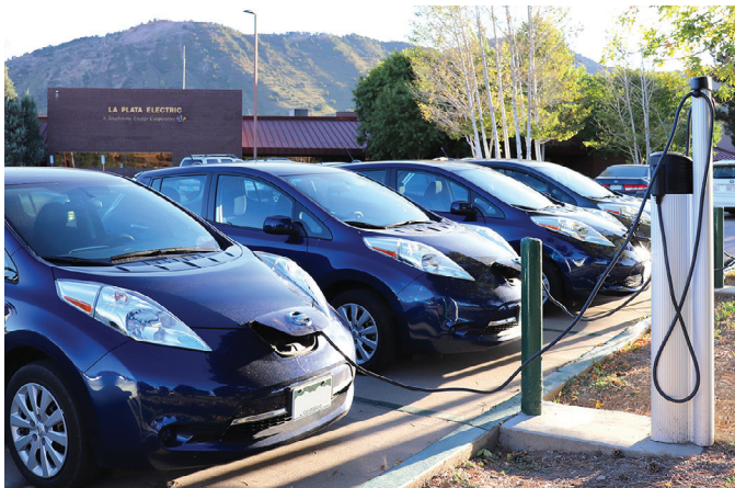
La Plata Electric Association's office in Durango features four ChargePoint Level 2 charging stations at 45 Stewart Street (Bodo Park), Durango, CO 81302.
